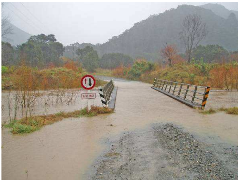
Figure 19: The effects of rain and flooding near Tolaga Bay, June 2009.
