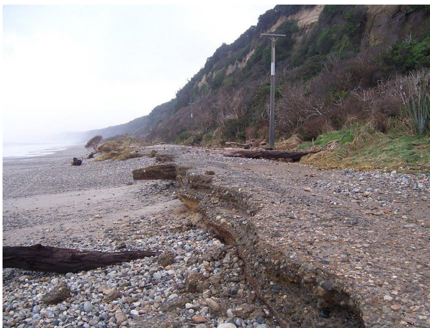
Figure 7-9: Coastal erosion of the Papatotara Coast Road along Te Waewae Bay (2007). Credit: Environment Southland.
