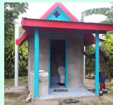
Completed ecoVIP2 (See KoroSan #6)
