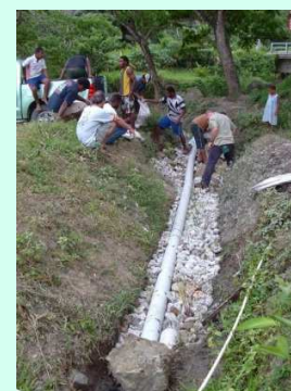
Constructing small wetland treatment area for grey water in drain to river
