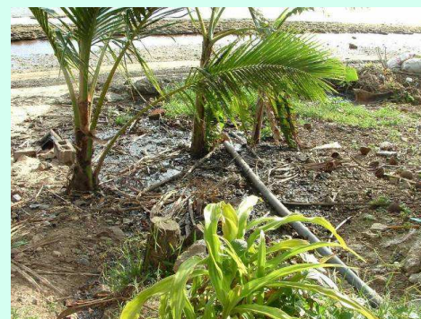
Septic discharge leaking onto beach and into lagoon.
