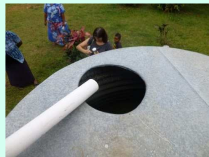
The lid for the water tank has fallen into the water tank.
