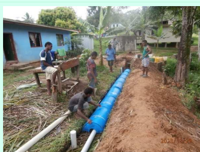
Waste water trench with half drums covering pipe.
